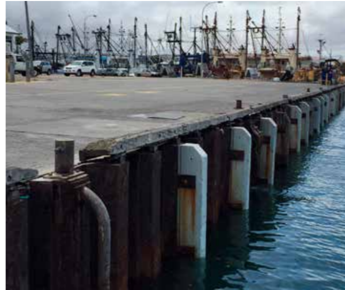
Existing wharf infrastructure is showing signs of deterioration and an upgrade is required
