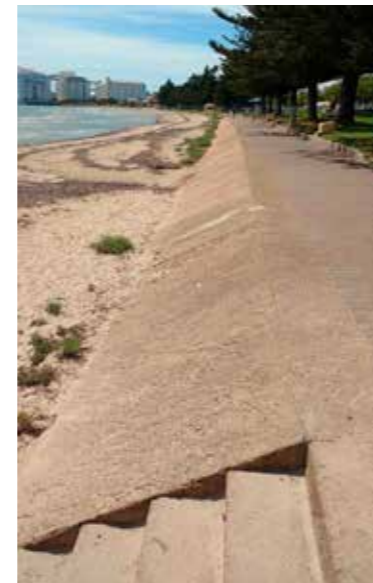
The existing sea wall shows signs of deterioration and allows sand movement + storm surge waves up onto the foreshore.
