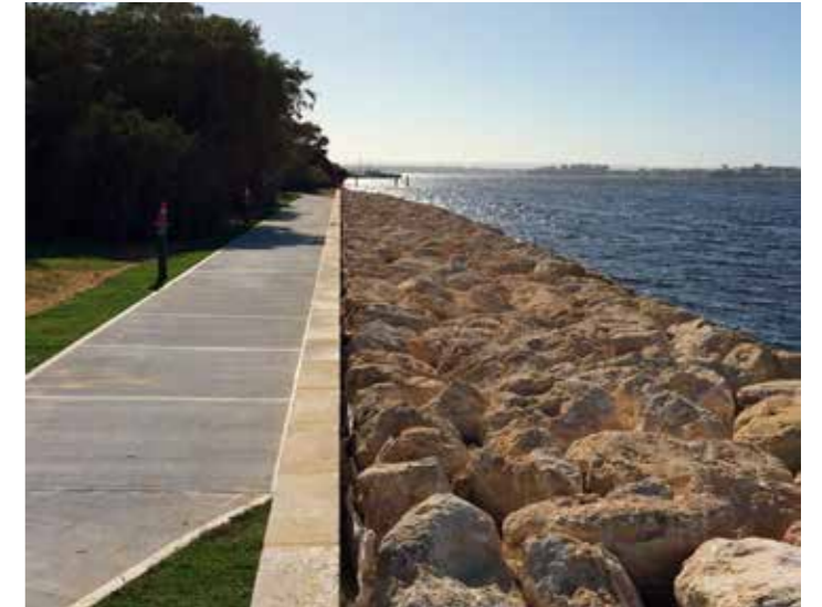
New rock revetment will enable the extension and widening of the Parnkalla Trail along to a formalised car park area.
