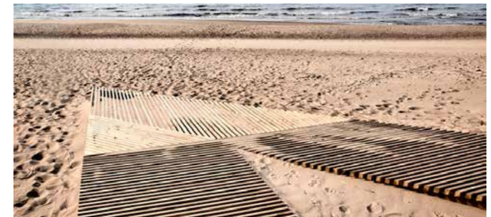
Timber slats to beach around Jetty to allow all abilities access to water.
